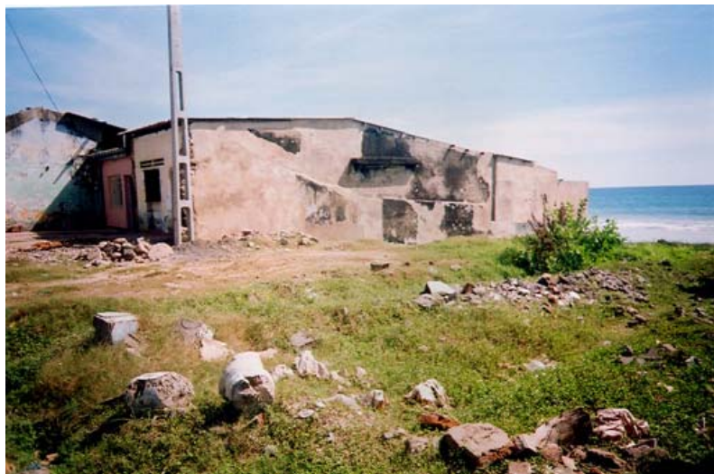
Photo 11: Illegally Reconstructed Houses in the New Buffer Zone
