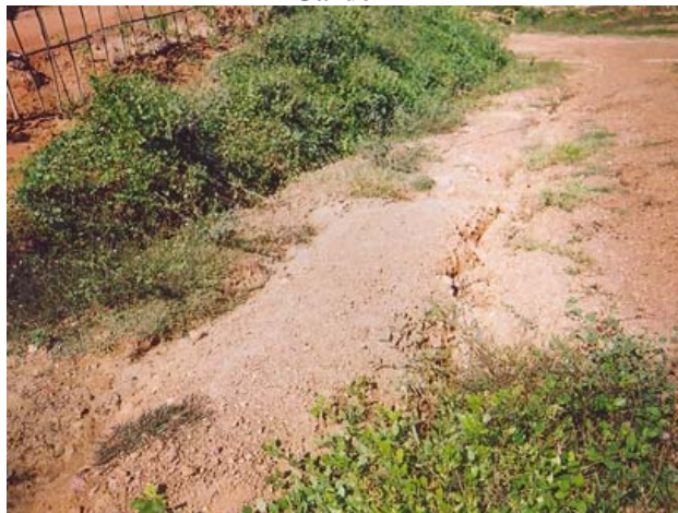
Photo 15: Damaged Gravel Access Roads at Tea Garden
