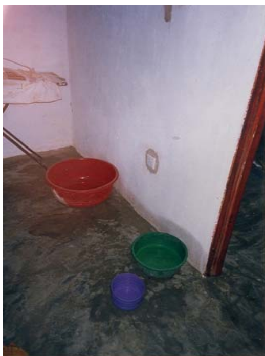
Photo 12: Water Leaking from the Roof of a House at Katupolwaththa
