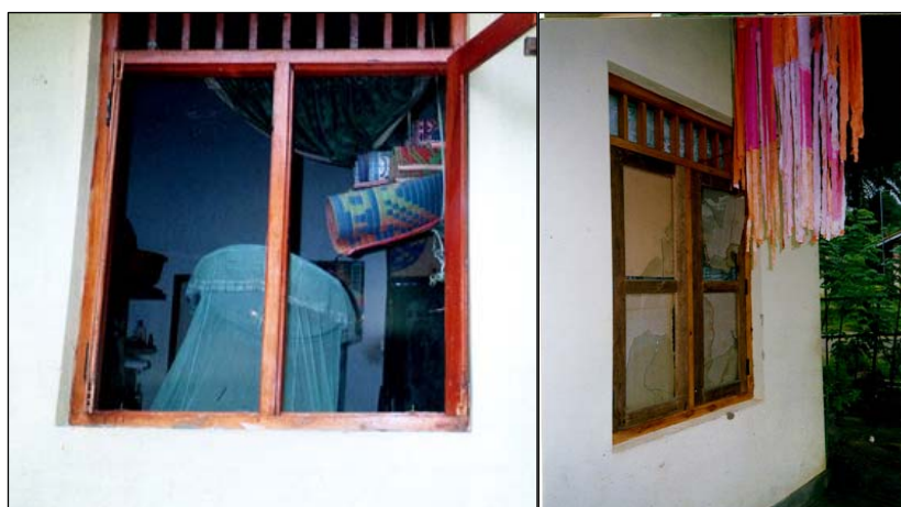
Photo 20: Windows of a Damaged House as a Result of Physical Conflict between Old Villagers and Katupolwaththa Settlers.
